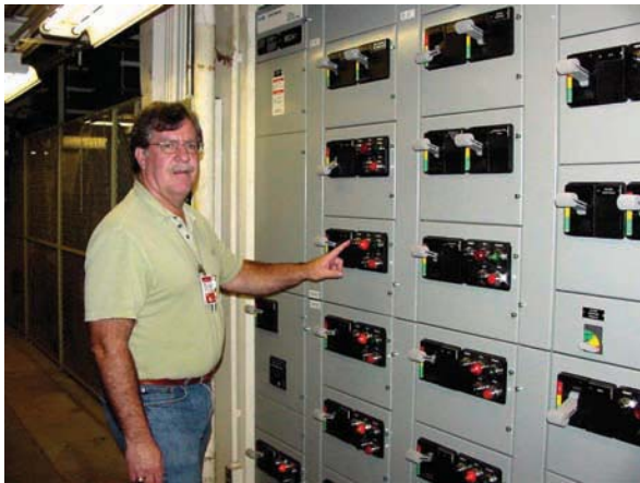
FIGURE 1: Operations Electrical Engineer Dennis Brady inspects the status indicator on a newly installed Motor Control Center.
