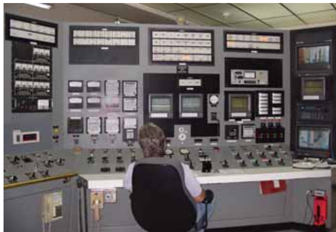
Operator Richard Beasley at the control console with refurbished displays.
