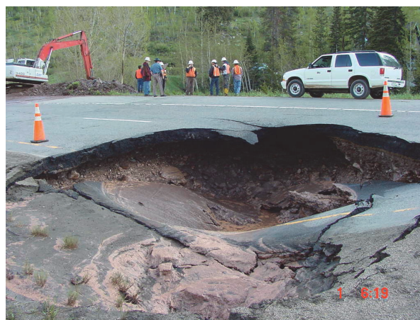
Figure 2. Photo. Vail Pass culvert failure.
