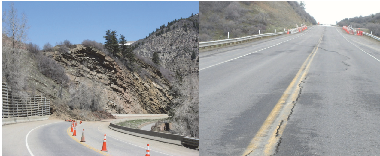
Figure 8. Photos. Examples of mobility loss and pavement distress from landslides.
