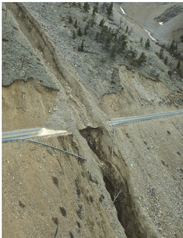
Figure 3. Photo. Debris flow damage on Beartooth Pass.
