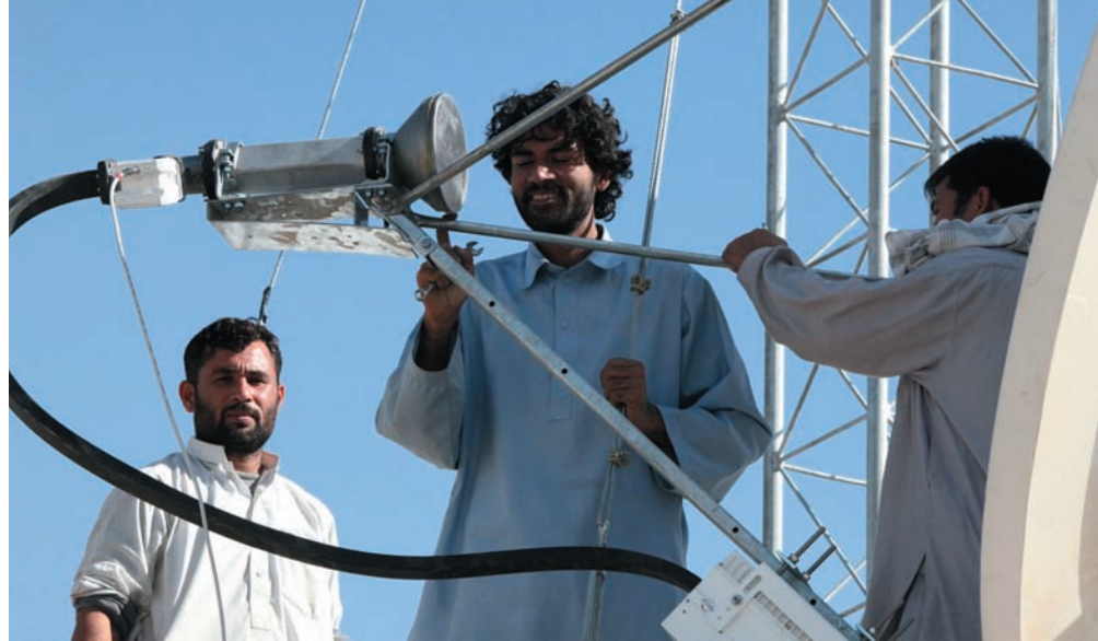
Local Afghan contractors install a satellite dish to the new cellular telephone tower at the Musa Qa'leh District Center, Afghanistan, Oct. 19, 2010. The tower is being built to equip a satellite dish that will provide cellular communication for the local people of Musa Qa'leh. (U.S. Marine Corps Photo by Lance Cpl. LaMarcus O. Adkins/Released)
