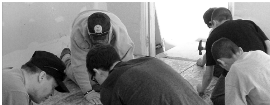
NAILED IT: Volunteers from the Colorado Springs Field Office and local Office of Personnel Management put down new raised flooring while converting a garage into living quarters for a disabled veteran.
