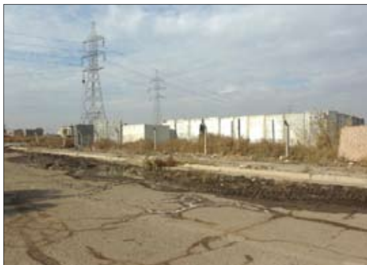
The future site of an electric power substation in the Saha neighborhood of southern Baghdad. The electricity provided by the substation is an example of the essential services the additional security provided by Sons of Iraq will allow for the citizens of the region.
