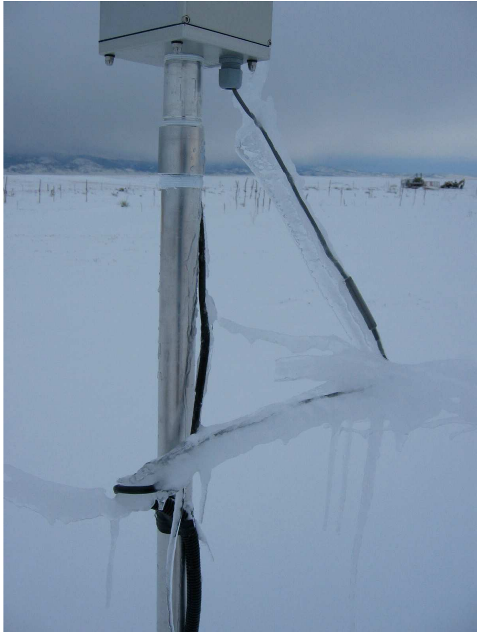
Figure 15. An example of how accumulated winter ice on exposed, unprotected wiring and cables can cause problems. Armored conduit protects wires from ice damage as well as hungry wild animals who chew on them.
