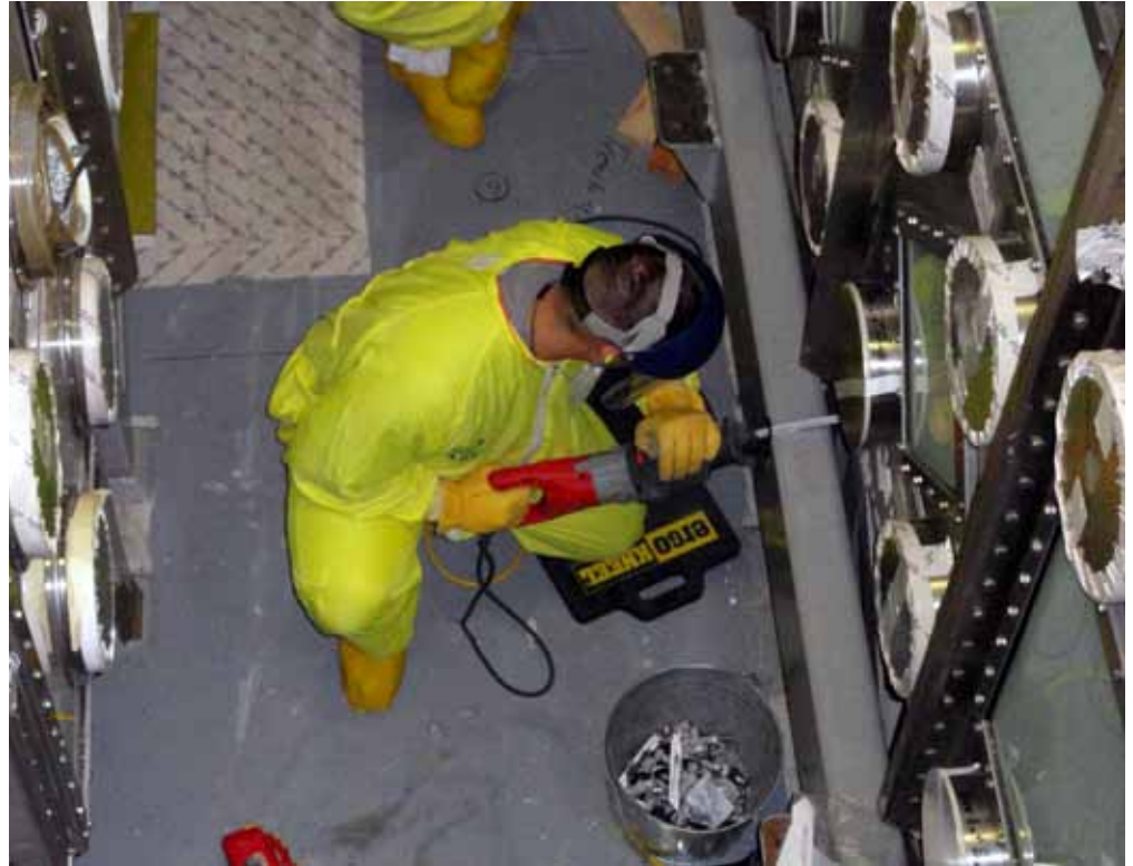
An ironworker cuts one of the steel seismic stabilization beams surrounding HC-230C-3, an oversize glove box in Room 230C at the Plutonium Finishing Plant. After the beams were removed, workers were able to continue dismantling other glove boxes that were once part of the Remote Mechanical C process line.
