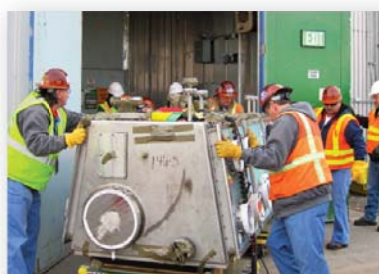
Accelerated demolition preparations will allow PFP and U Canyon to be demolished ahead of schedule
