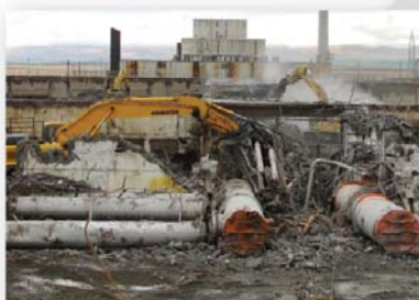
Removing buildings and debris sites and remediating waste sites significantly reduces the active area of cleanup, including the area of cleanup around the K East and K West reactors
