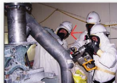
Removing excess and ancillary facilities that are no longer of service reduces future surveillance and maintenance costs
