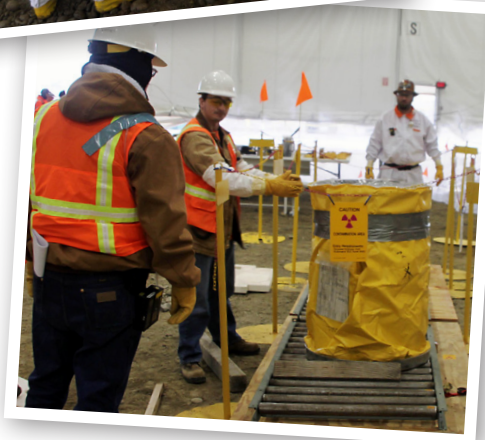
A drum of waste, wrapped in protective plastic, is readied for processing adjacent to the 12B burial ground.
