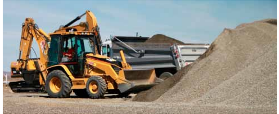
Workers move fill dirt at the future site of the 200 West Groundwater Treatment Facility.
