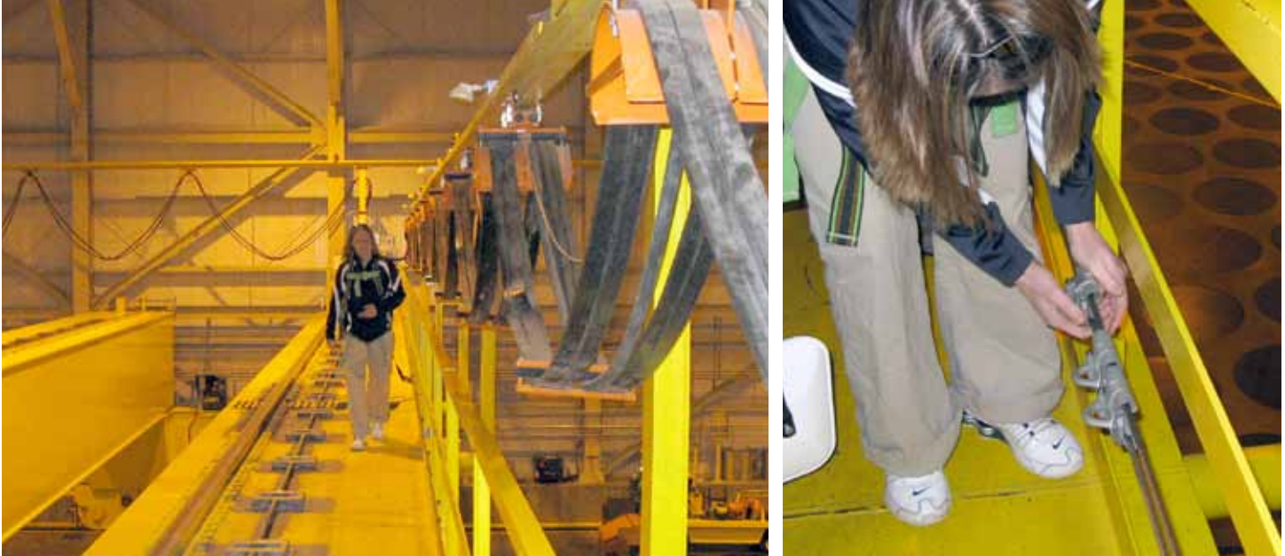
Kami Johns, a trainer at the Canister Storage Building, demonstrates the new fall protection system on the multi-canister over-pack handling machine (left). As Johns walks across the beam, she is protected from a potential fall by wearing a harness that is secured to a traveler (right). The new double-cable fall protection system allows workers to safely walk across the beam to access the turret wherever it is parked.
