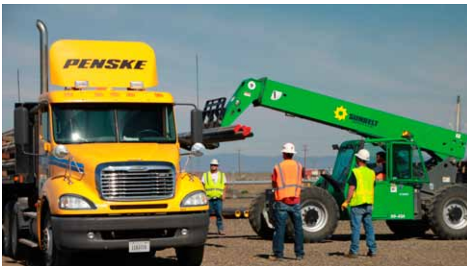
Workers move piping at the future site of the 200 West Groundwater Treatment Facility.
