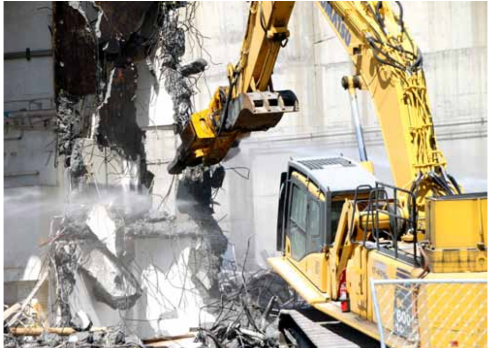
CHPRC D&D workers are demolishing the 224-U building (above). The building is one of three U Plant ancillary facilities currently undergoing demolition in preparation for the ultimate demolition of the U Plant processing canyon.
