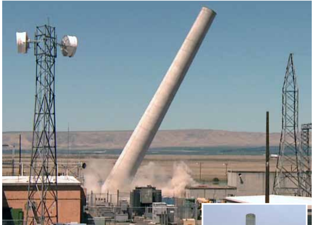
The 116-KE stack falls on July 23 after explosive demolition techniques are used to bring it down. Workers have been clearing the stack and other structures that are no longer in service from the 100K Area.
