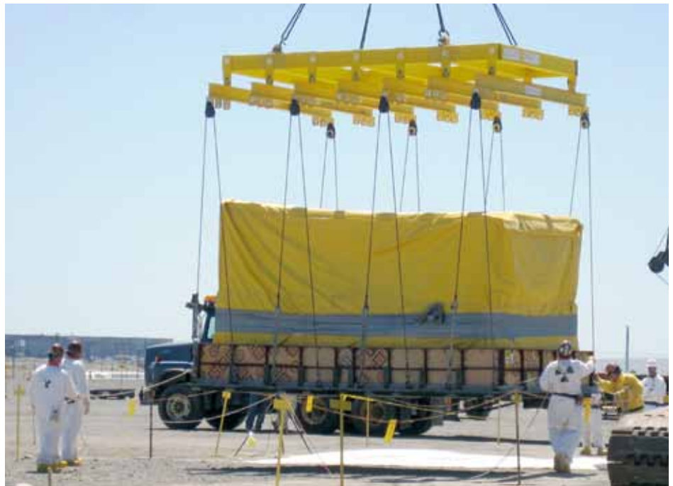
Members of the waste retrieval team watch as Box 3 is lifted from Trench 17 and placed on the ground where workers can finish building another box around it. Before it was lifted, the deteriorated box was enveloped in a layer of protective material and placed on a base that supports the box while it is moved.
