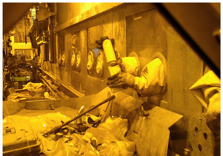
An example of the interior of a WRAP glovebox (taken prior to implementing HexArmor gloves) where workers operate through gloves and remove prohibited items from TRU waste drums. The HexArmor Overglove is designed to fit over the glovebox glove, providing cut/puncture resistance.
