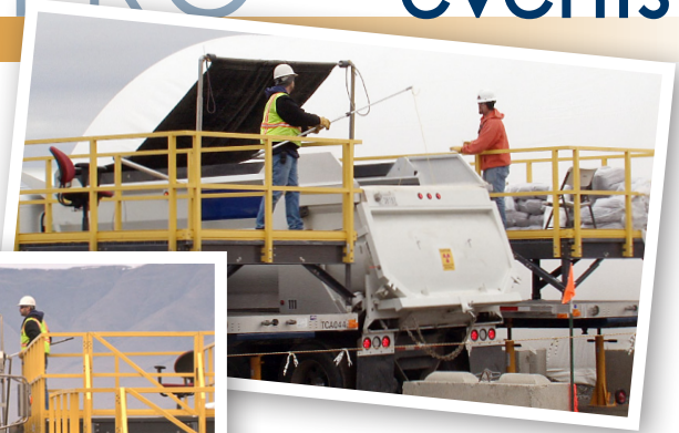
The first set of platforms is in use at the BC Control Area.
