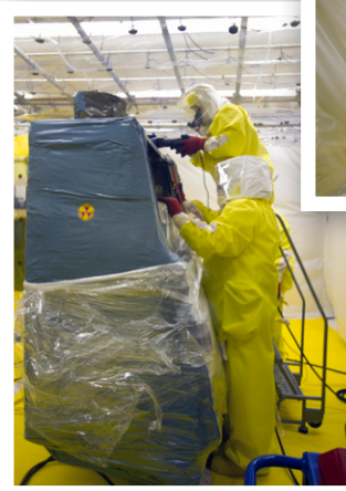
Workers cut up a glovebox. Gloveboxes are large, sealed pieces of equipment — ranging in size from 35 to more than 1,200 cubic feet — that once supported plutonium production and processing.
