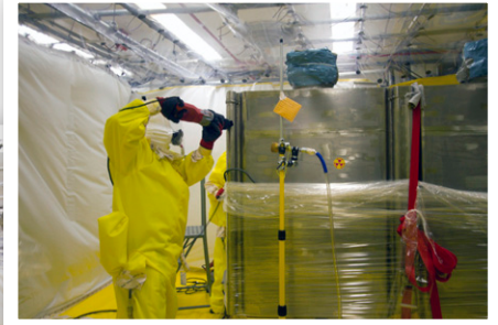
A worker cuts up or “size reduces” a glovebox so it can be packaged for shipment and disposal
