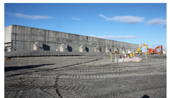
The site of the ancillary facilities after demolition outside of the U Plant canyon
