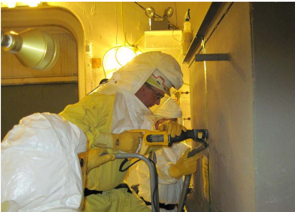
Workers remove the east end of a highly contaminated tank in the Criticality Assembly Room of the 209-E Critical Mass Laboratory to provide access to two storage tanks as part of demolition.
