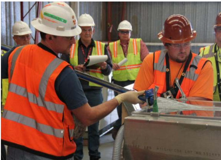
Crews demonstrate procedures on a “cutting shroud” that would be used to tackle the last major hazard in the 209-E Critical Mass Laboratory prior to demolition -- highly contaminated tanks that had to be cut up and removed before the building could be demolished.
