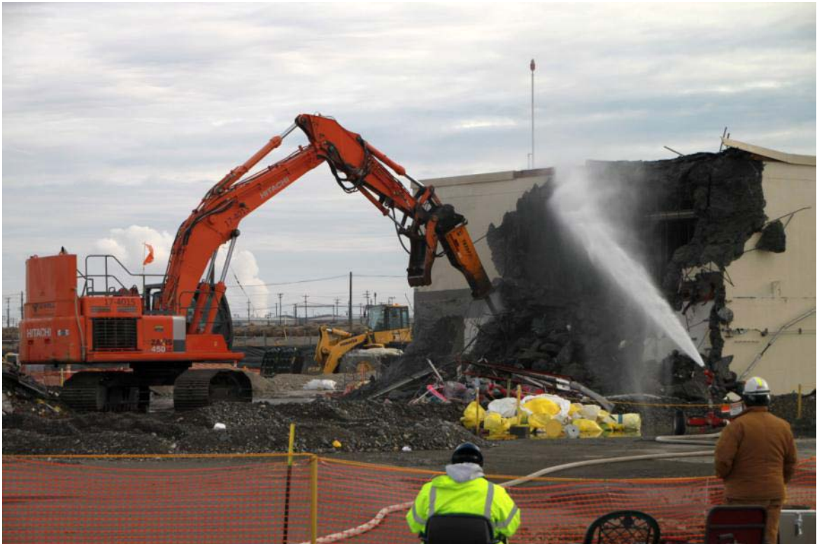
CH2M HILL workers tear away at the 5-foot-thick concrete walls of the 209-E Critical Mass Laboratory. The laboratory was run by Battelle for years to identify controls for criticalities, the term used for the dangerous condition when fissile material can sustain a reaction by itself. The facility housed experiments to test the criticality limits of uranium and plutonium solutions.
