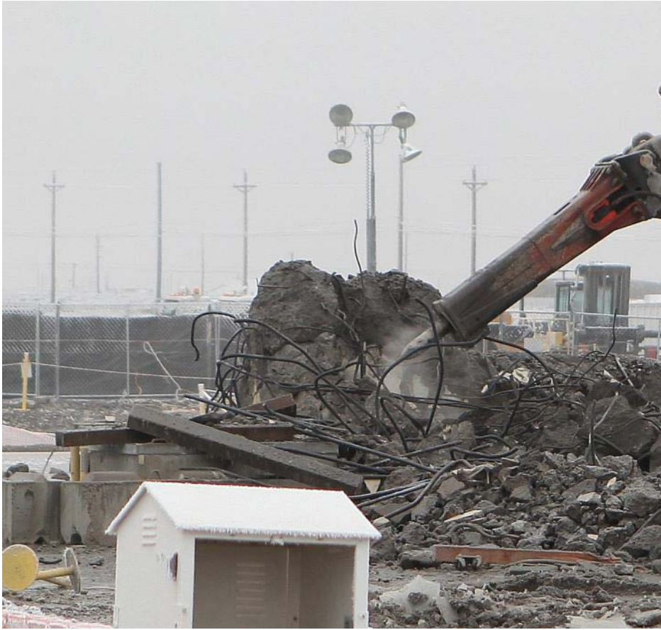
CH2M HILL crews finish demolition of the 209-E Critical Mass Laboratory. The project took two years to safely prepare the nuclear facility and workers for the demolition.
