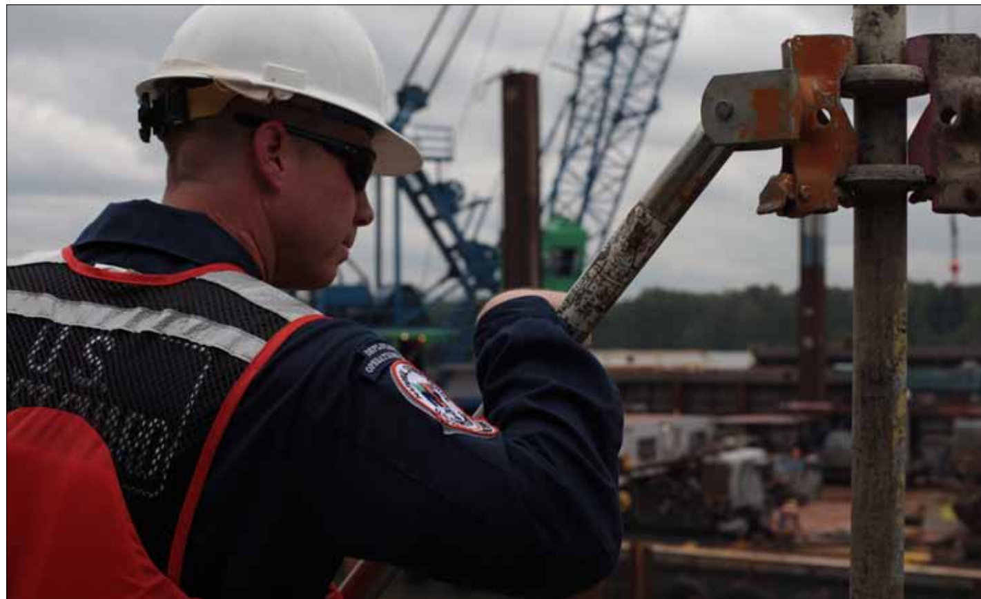
Petty Officer 1st Class Michael Shannon, a marine science technician from the Pacific Strike Team, stands safety watch over the 431-foot flat deck barge Davy Crockett during disassembly operations on the Columbia River, June 8, 2011.
