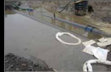
Pipeline repair was halted for days when heavy rain displaced sorbent boom and pads.
