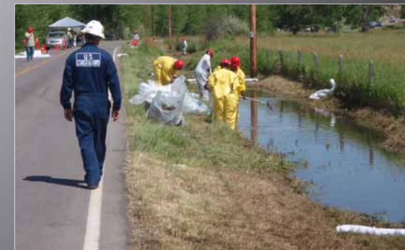
A strike team member monitors cleanup efforts at the Exxon Silvertip Pipeline Spill near Laurel, Mont., July 8, 2011.
