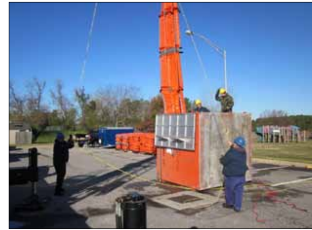
Contractors install new foam-filled boom into boom containers in Portsmouth, Va. U.S. Coast Guard photo.
