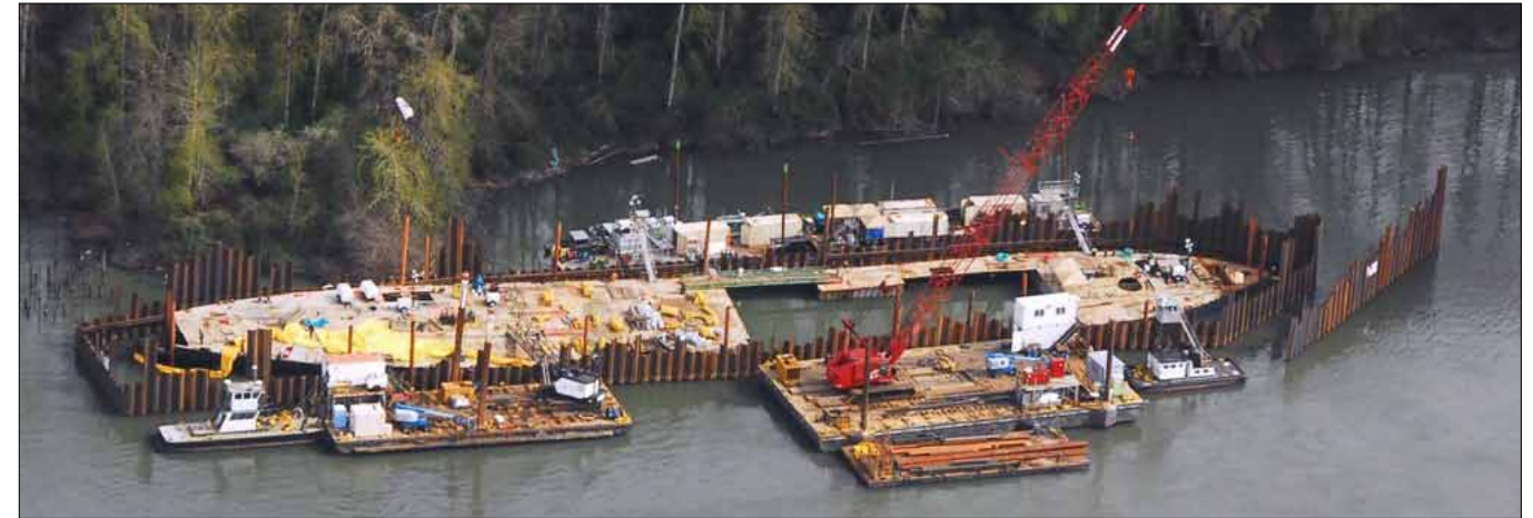
The barge Davy Crockett sits enclosed by a cofferdam in the Columbia River near Camas, Wash., April 18, 2011. The cofferdam holds pollutants as crews work to dismantle the barge and remove it from the river. Photo provided by Davy Crockett Response Unified Command.
