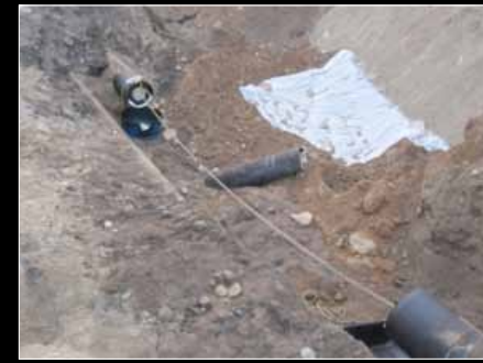
The damaged section of the pipeline is prepped for a temporary patch.
