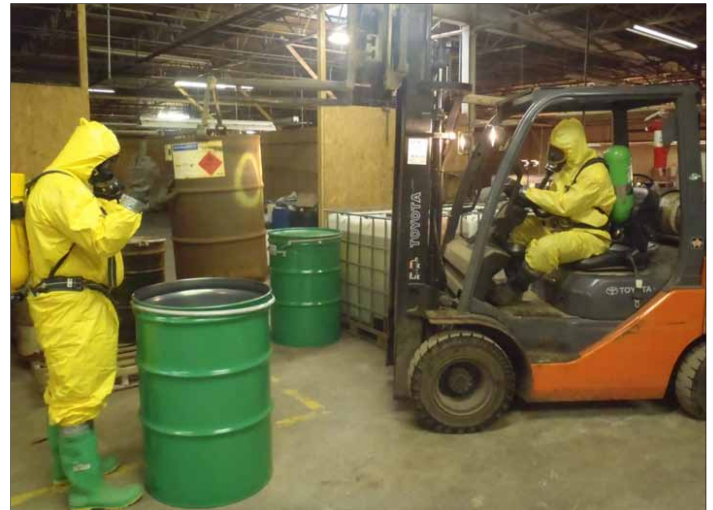
Contractors at the BioTech facility work to remove hundreds of drums containing hazardous materials from the facility, Feb. 10, 2011. Many of the containers were damaged and posed a threat to surrounding communities.
