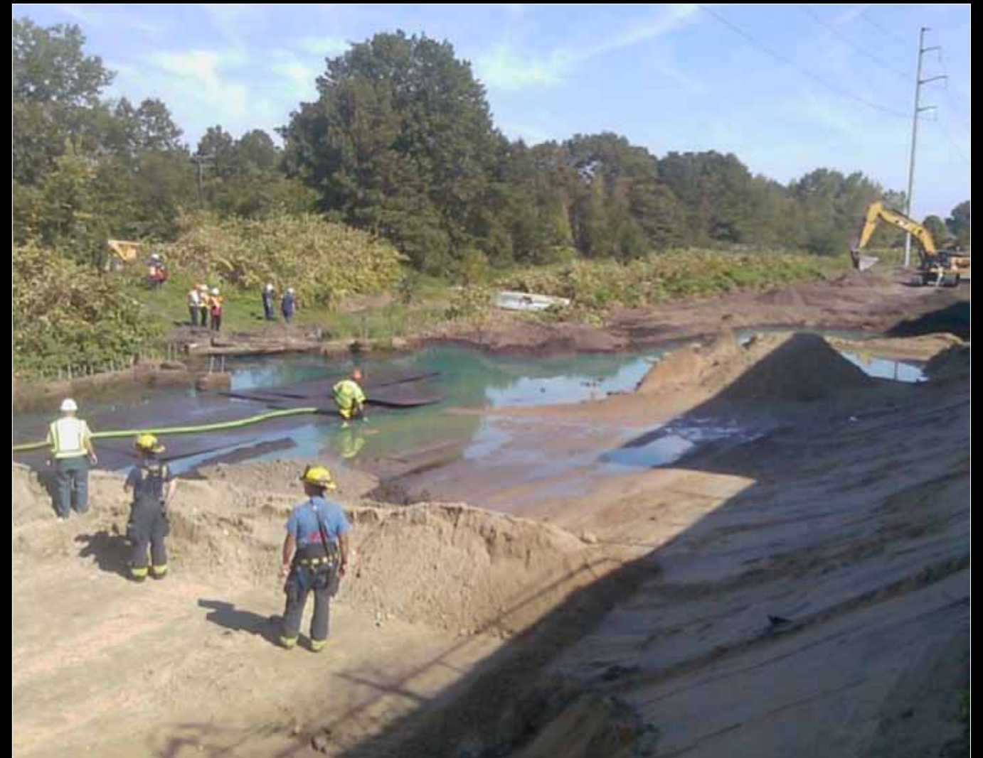
Contractors conduct cleanup operations at the Capital Terminal facility, Sept. 4, 2011 after an estimated 70,000 gallons of No. 2 low sulfur diesel fuel leaked from a ruptured pipeline. U.S. Coast Guard photo.
