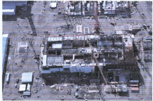
Figure 2. The Pretreatment Facility
