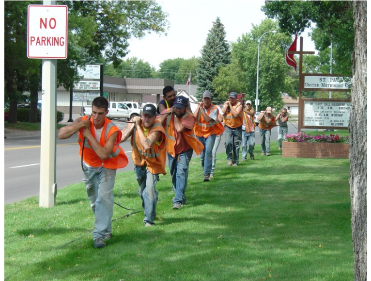
Workers drag fiber to be laid as part of Daktel's 100% Fiber-to-the-Home network, the largest in the United States
