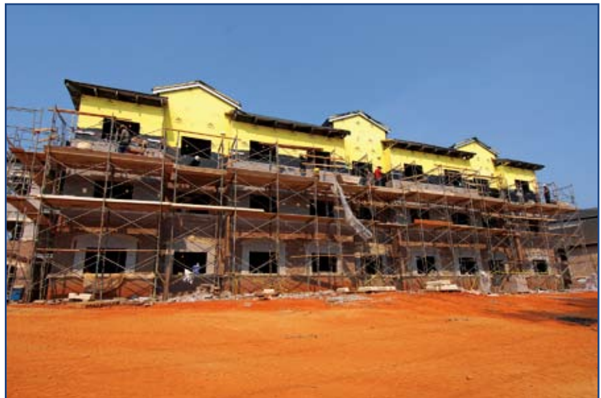
Shaw AFB is investing in environmentally friendly dormitories that are expected to meet LEED Silver certification criteria. One of the technologies in use is a geothermal well for heating and cooling.
