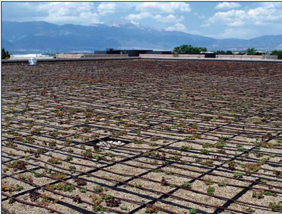
Vegetative roofs can help cut down on utility bills as well as rainwater runoff by insulating the roof from the heat of the sun and capturing the rainwater for the plants. The Air Force is testing the concept on an administrative building at Peterson AFB.
