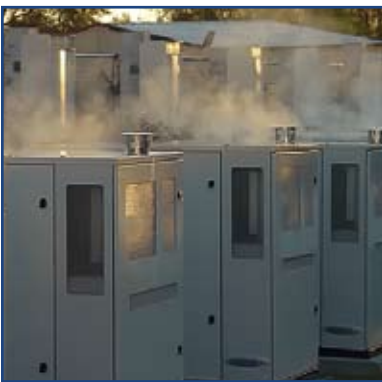
Top: Dyess AFB uses an effluent pond as a cooling tower for the base ice plant, which provides cooling for 14 buildings.
