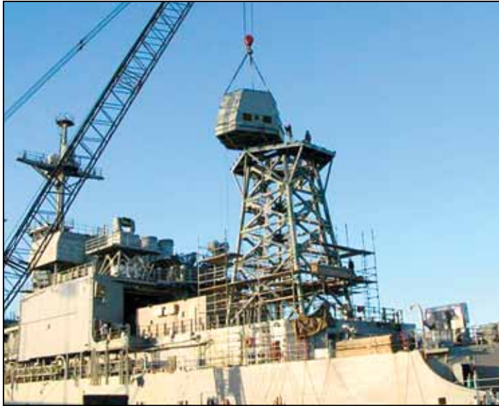
Figure 3. MFR Antenna Shelter Being Mounted on Tower Onboard SDTS
