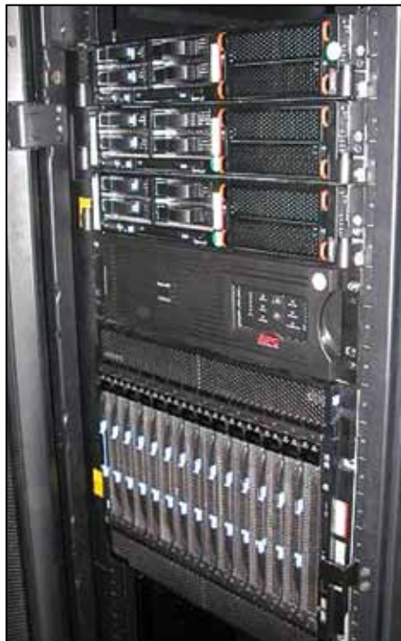
Digital Signal Processor and Radar Control Processor (IBM Blade Servers)
