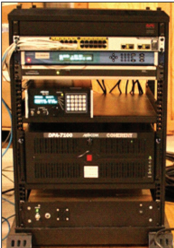
Figure 2. Remote Location Equipment
