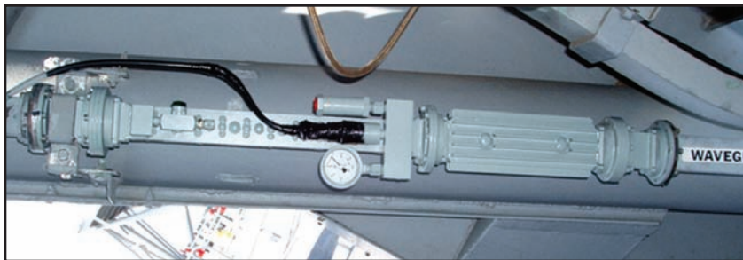
Figure 2. Sulfur Hexafluoride (SF6) Gas-Filled Filter Installed Aboard USS Tarawa
