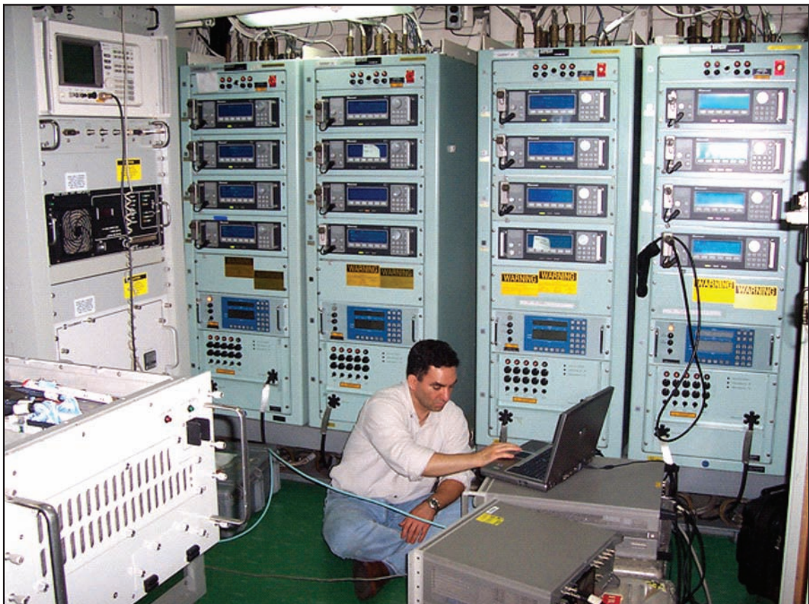
Figure 6. Dahlgren engineers conduct an electromagnetic assessment in a radio transceiver room aboard the amphibious assault ship USS Iwo Jima (LHD 7).
