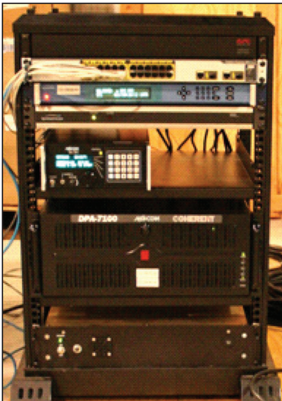
Figure 2. Remote Location Equipment
