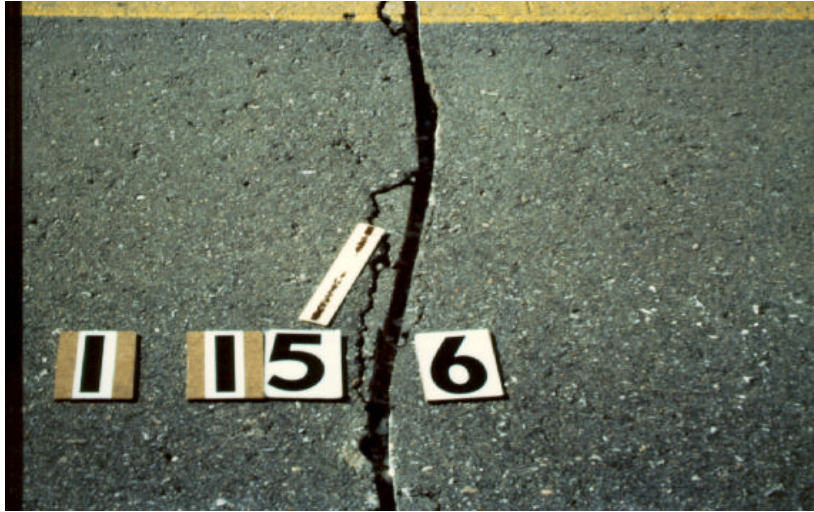
Figure 17. Crack segment missed by cutting equipment.
