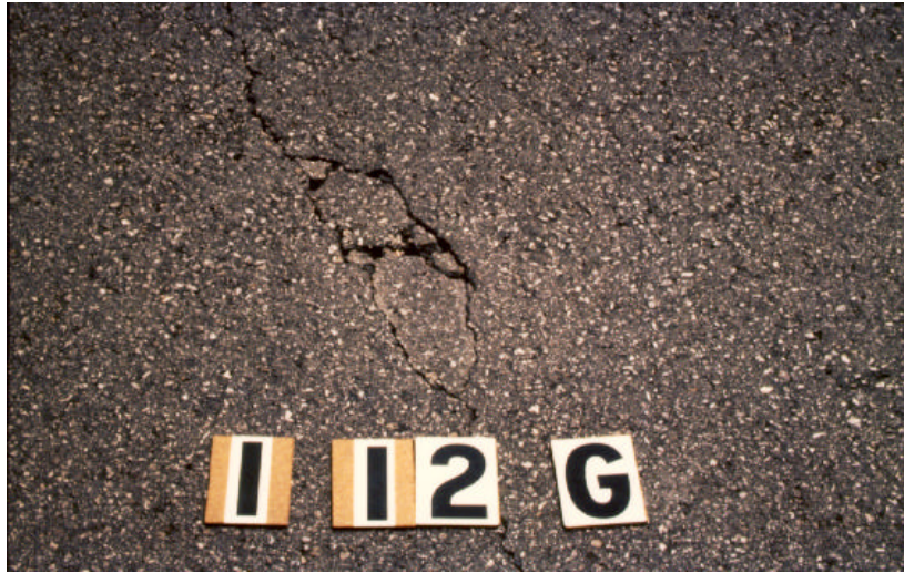
Figure 18. Primary crack accompanied by secondary crack.
