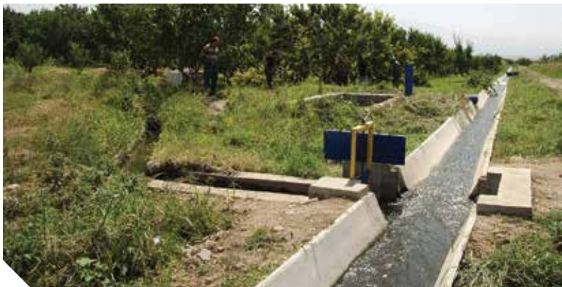
Margarita and her neighbors' three-kilometer canal is just a small segment of approximately 220 kilometers of tertiary canal rehabilitated under the MCC compact.
