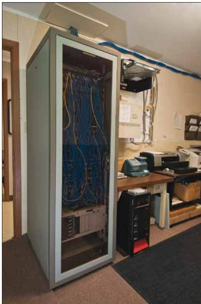
The equipment room at a USDA Service Center office
