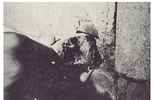
FIGURE D-4 Probing Cracks in Concrete Wall for Khapra Beetle
