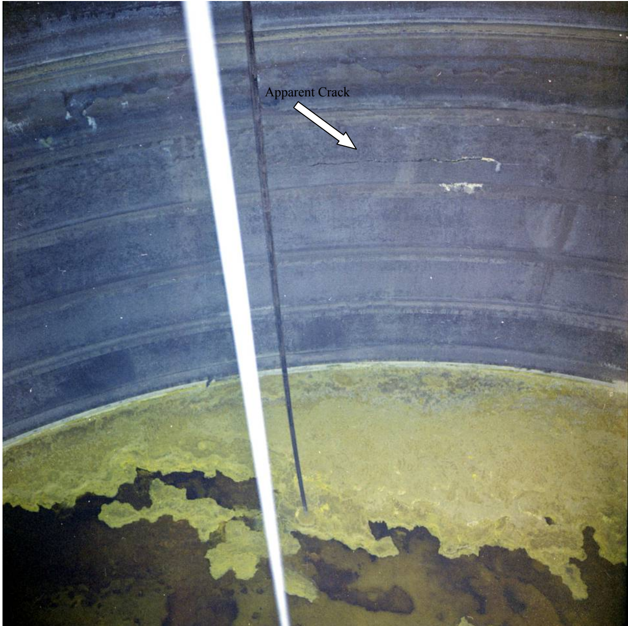
Figure 5.7-3. Crack in Tank 241-SX-112 Sidewall at ~16-ft Elevation
