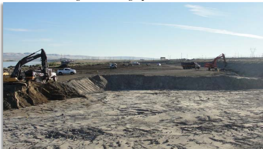
View toward the east of excavation and waste loading at waste site 100-K-63.
