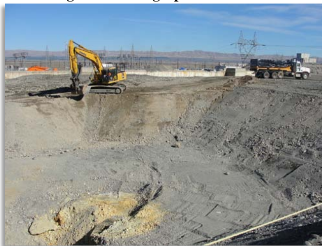
View toward the northeast of excavation and waste loading at waste site 120-KW-1. Note the large chemically-stained soil in the bottom-left side of the photo.
