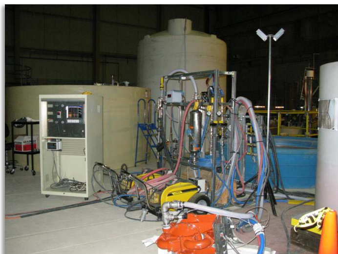
Test Top Retrieval System
