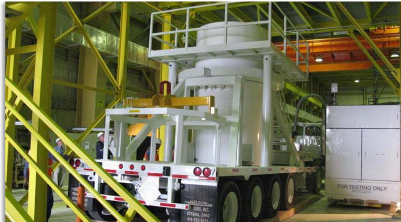
Sludge Transfer Storage Cask (STSC) Positioned at the Maintenance and Storage Facility
