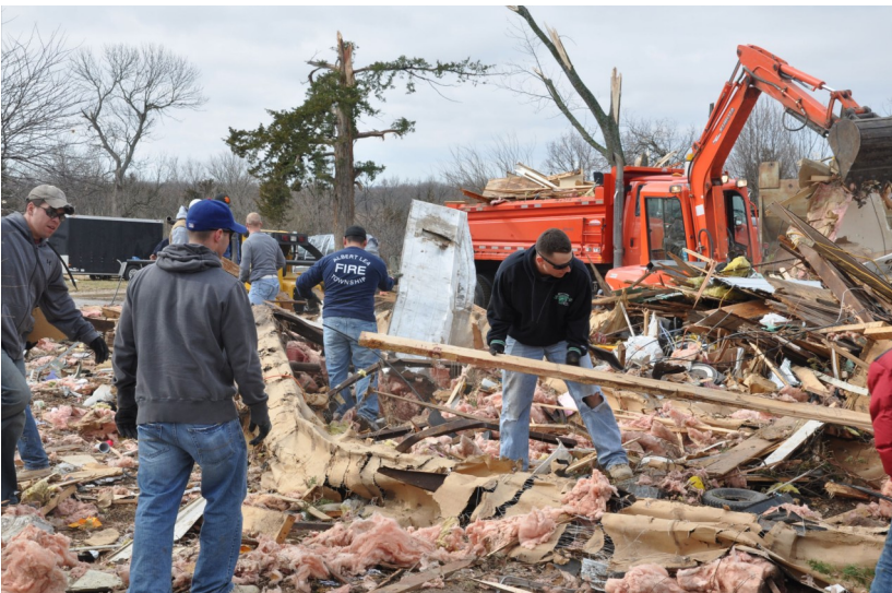
Harveyville, KS —SSG Hendricks and SPC Massari lift heavy beams that used to be part of a house during cleanup of Harveyville. (U.S. Army photo by Spc. Brandon Cunliffe-Owen, 2nd AAB, 1st Inf. Div., USD-C)
