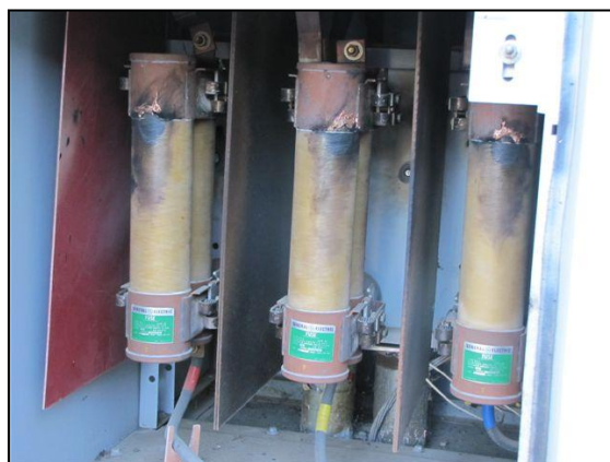
Blown 150 amp, 15,000-volt fuses at Maintenance and Storage Facility
