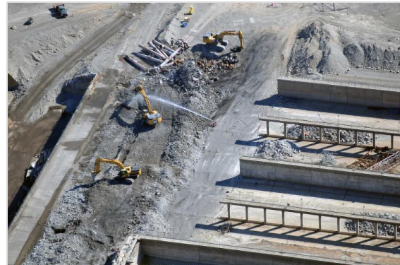
183KE Water Retention Basin
