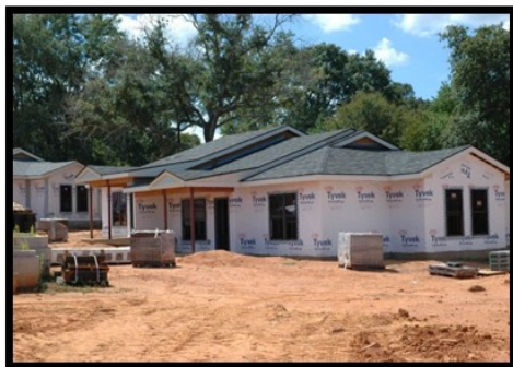
The housing authority’s newest locally-owned development under construction. The units were built to be energy efficient and withstand high winds.
