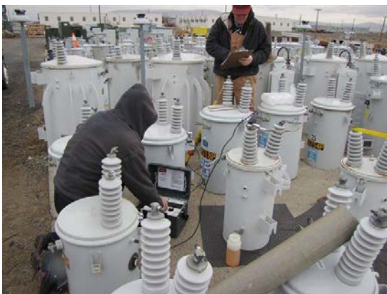
Electrical Utilities tests pole mounted transformers for upcoming projects
