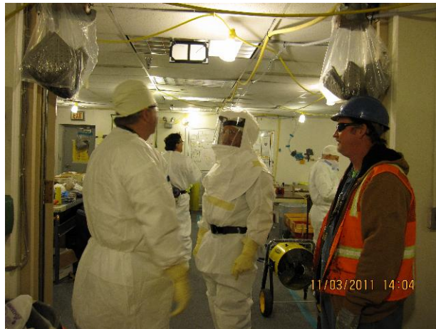
Painters ready to apply a lock-down material to highly contaminated Rad Zone at 209-E in preparation for demolition.
