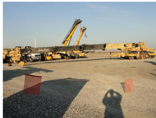
Fleet troubleshoots repairs on Grove 110 ton crane in the radioactive material area
