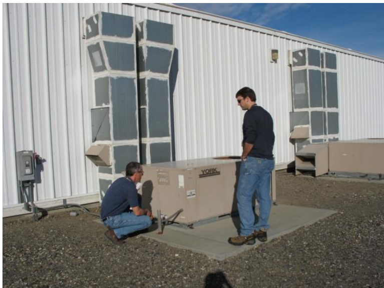
Verifying energy data of an HVAC unit in the 200 West Area.
