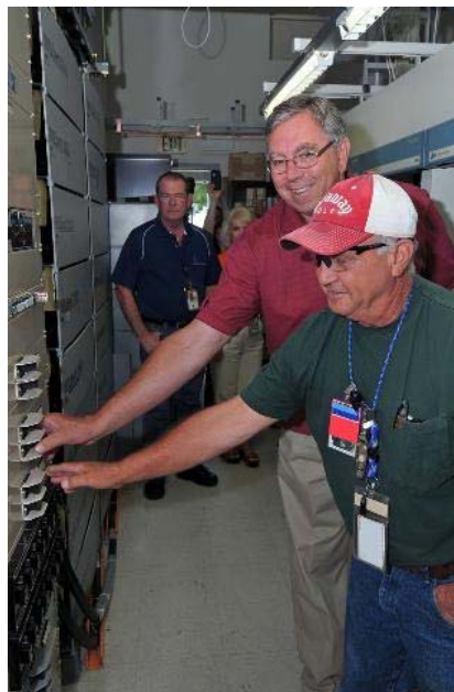
5ESS Switch Powered Down
