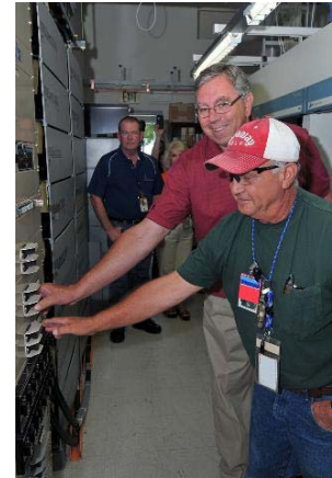
5ESS Switch Powered Down
