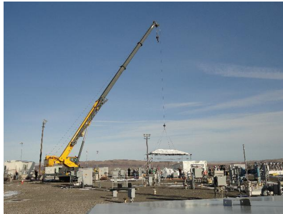
Crain & Rigging personnel relocate a containment tent to support pump removal at AN Tank Farm
