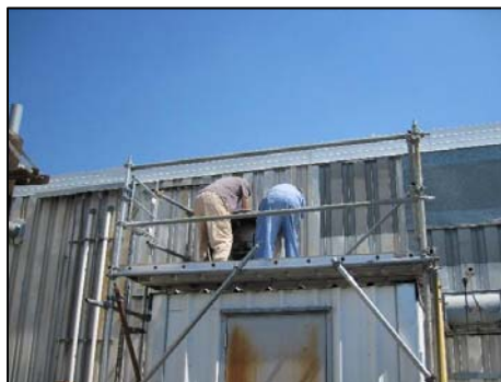
Installing a new fan motor to exhaust two fume hoods in 2101M Building
