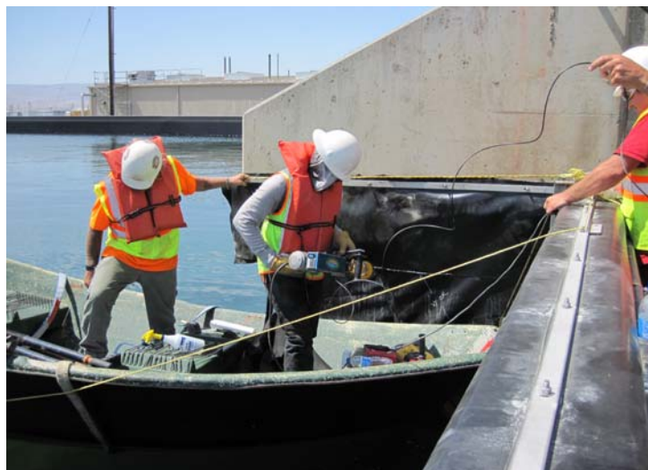
Completing the Last Construction Punch List Item on the Project L-311 "Raw Water Reservoir Relining"
