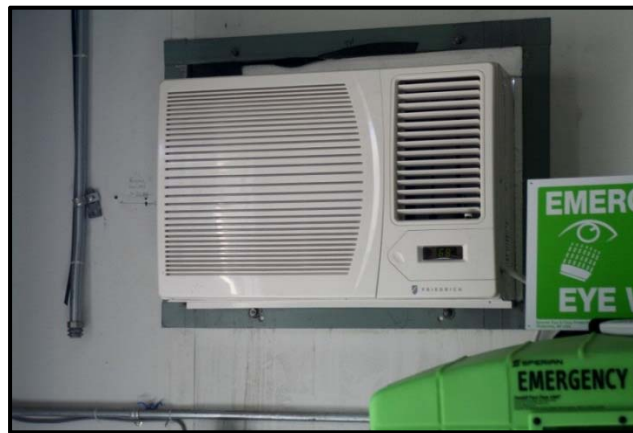
New AC Units installed
