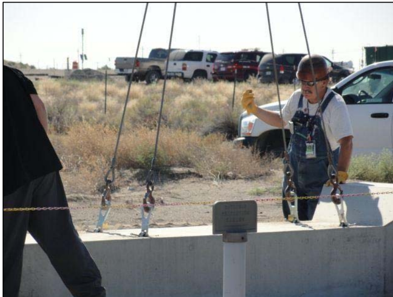
Crane & Rigging personnel staging hose barn for shielding hose in hose transfer lines
