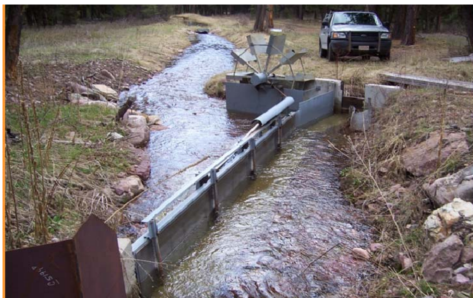
Figure 9. Fish screen installed to keep fish out of irrigation ditches
