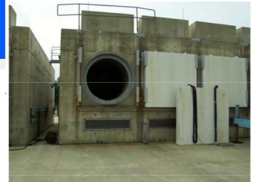
'Jones 2010.ppt', Calvert Cliffs Dry Fuel Storage and Industry Lessons Learned
