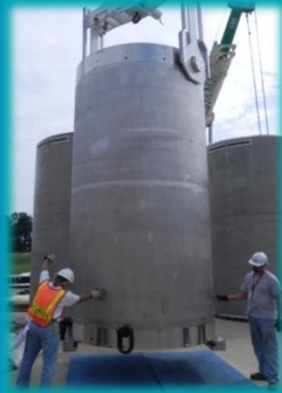
Transfer Cask At McGuire
