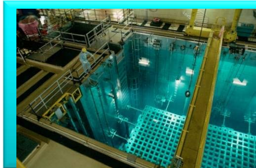
Spent Fuel Pool (on site)
