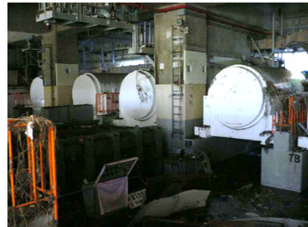
Figure II-2-56 Situation in Dry Storage Cask Facility
