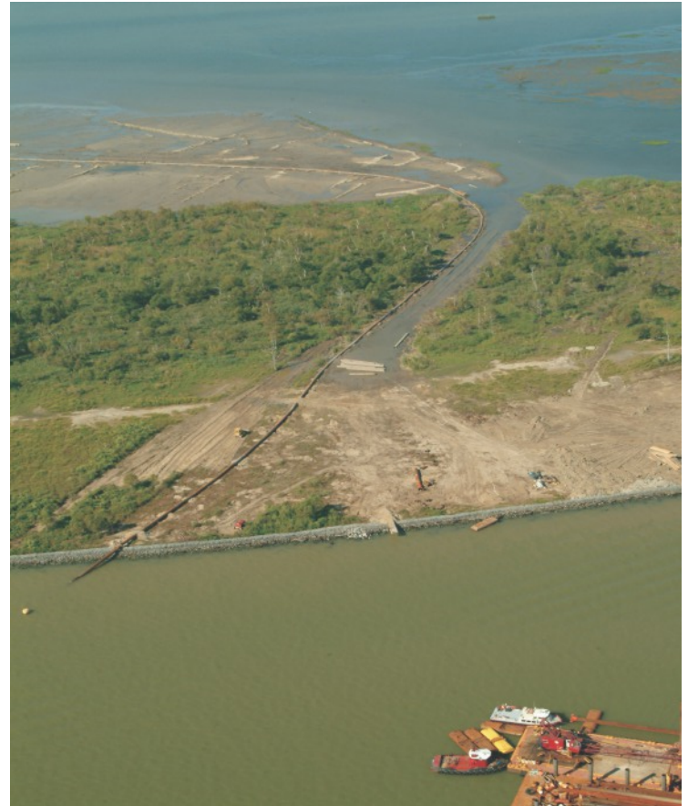
A dredge is being used to create marsh in the lower delta for the West Bay Sediment Diversion (MR-03) project. Work similar to this will take place during construction of the Benneys Bay project.
