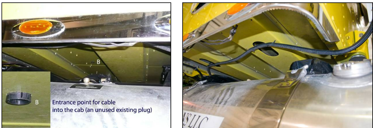
FIGURE 6 Routing of the Reader Ethernet Cable in the Truck Undercarriage
