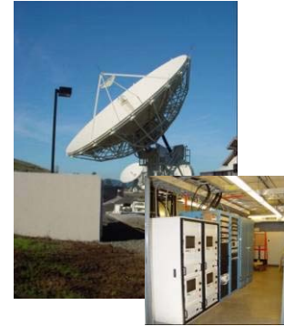
4 Ground Earth Stations
