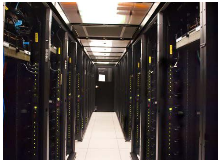
Figure 4 6. View of the RSF data center in the cold aisle (top) and from inside of the contained hot aisle (bottom) Photo by Dennis Schroeder, top: NREL/PIX 19219, bottom: NREL/PIX 17897
