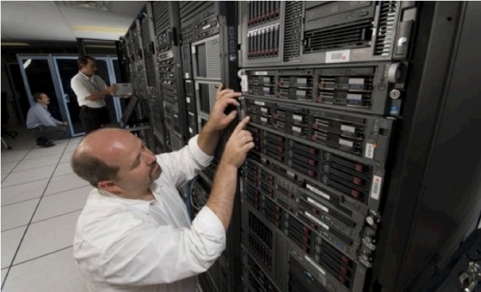
Figure 2 1. NREL's legacy data center Photo by Patrick Corkery, NREL/PIX 15885
