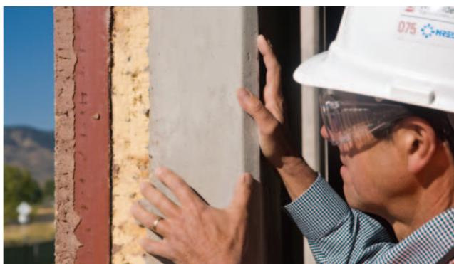
The precast panel's exterior keeps the weather out and helps regulate the interior temperatures. Photo by Patrick Corkery, NREL/PIX 16763
