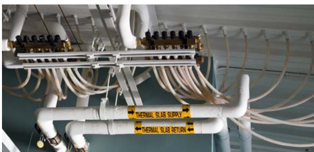
Forty-two miles of tubing run through the RSF ceilings to provide radiant heating and cooling. Photo by Dennis Schroeder, NREL/PIX 19443
