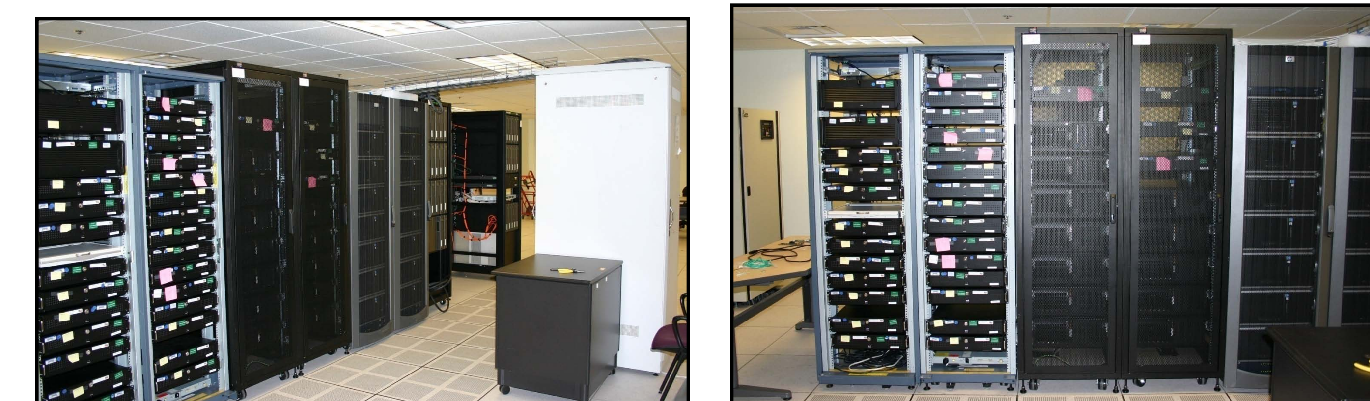
Current configuration of the DISC server room with seven racks in place.
